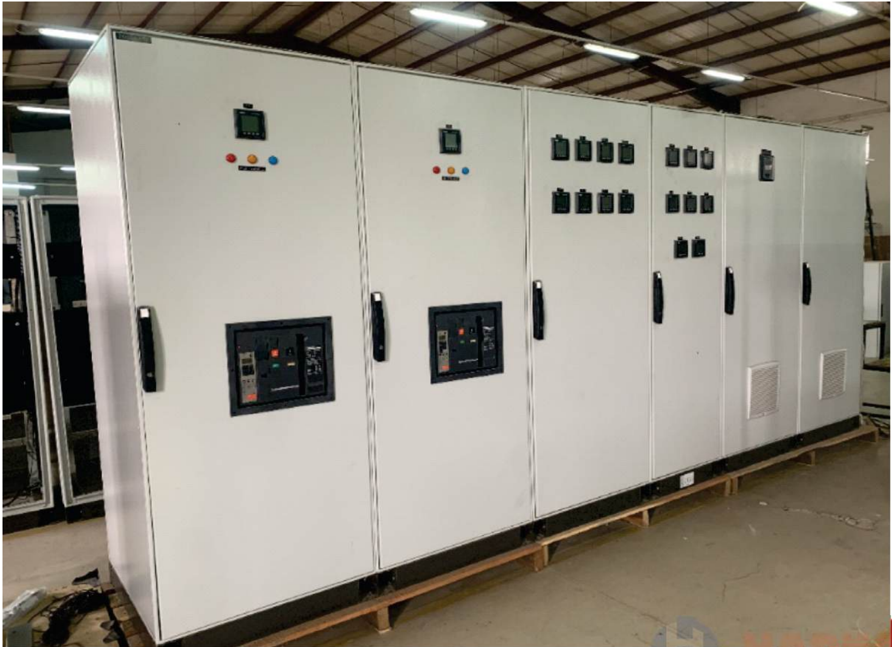
4000A Synchronization Panel
