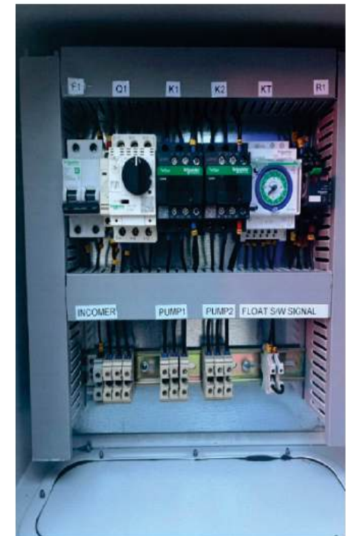
Starters for Pumps
