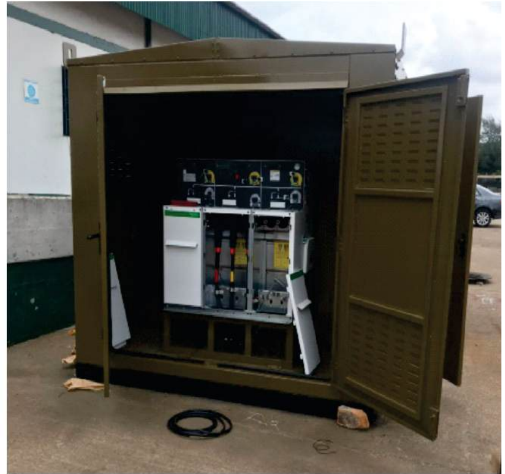
2500kVA 11kV Packaged substation (Transformer, 11kV SWG, LV Panel)
