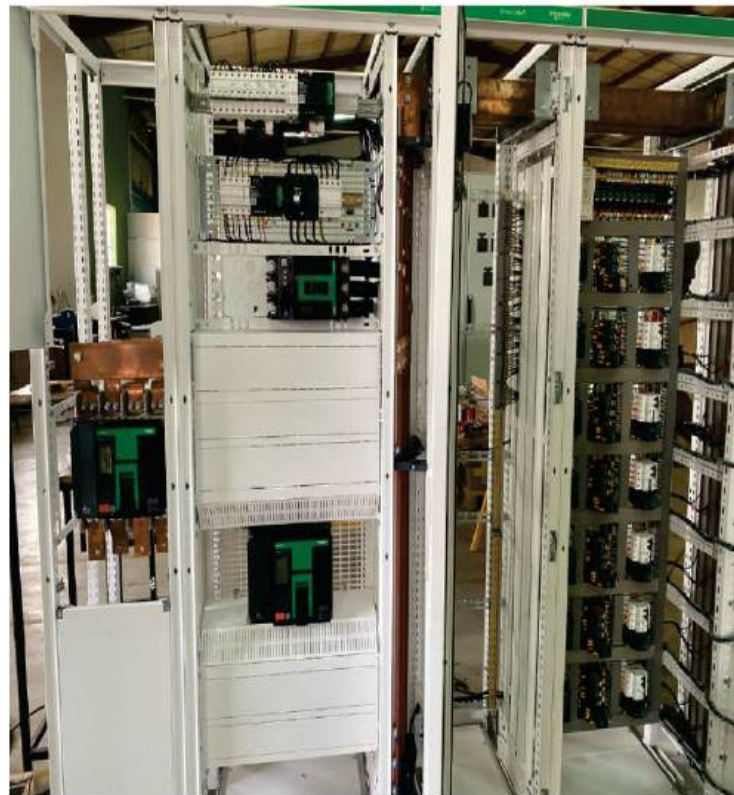
Motor control Center Panel
