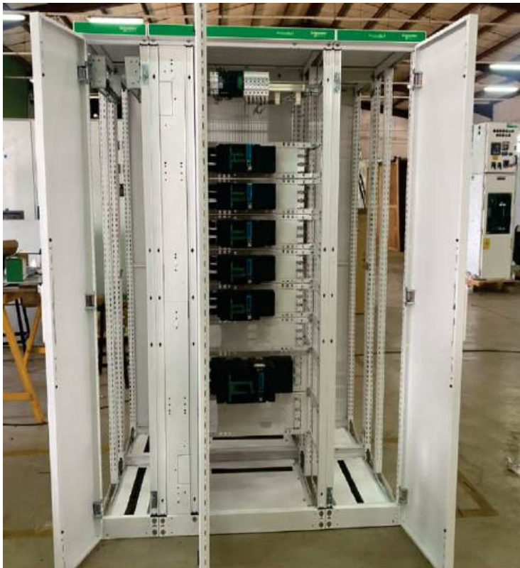
630A Distribution Panel
